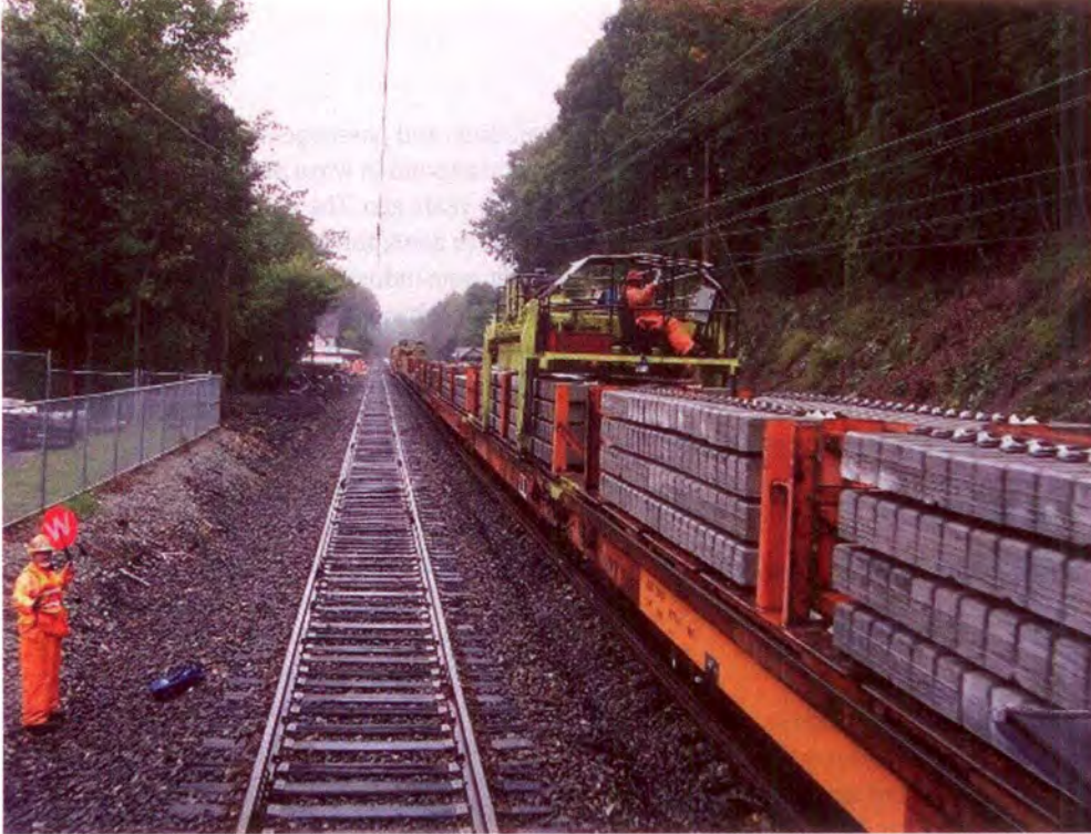
On Pennsylvania's Keystone Corridor, Amtrak made high-speed upgrades, including welded rail and trainloads of concrete ties.
